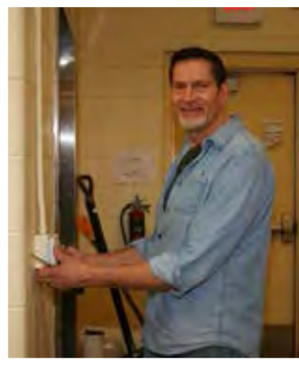
► Mark Sauers is repairing a light switch for the House of Peace. Mark joined the staff in July as Maintenance Director. He has professionally managed maintenance departments for several retirement communities.
