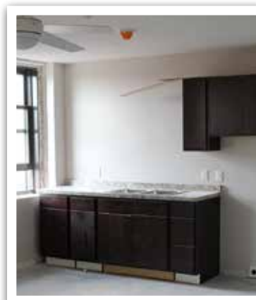
▲ Kitchen cabinets, lights, smoke and fire alarms were all being installed in August when this picture was taken. To see more current photos go to the St. Anthony's link on our website.
