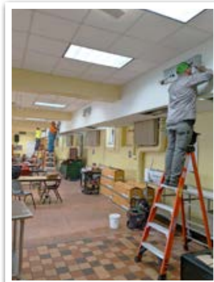
▲ St. Ben's Meal site: HVAC contractors install vents in the new drywall that encloses the system.
